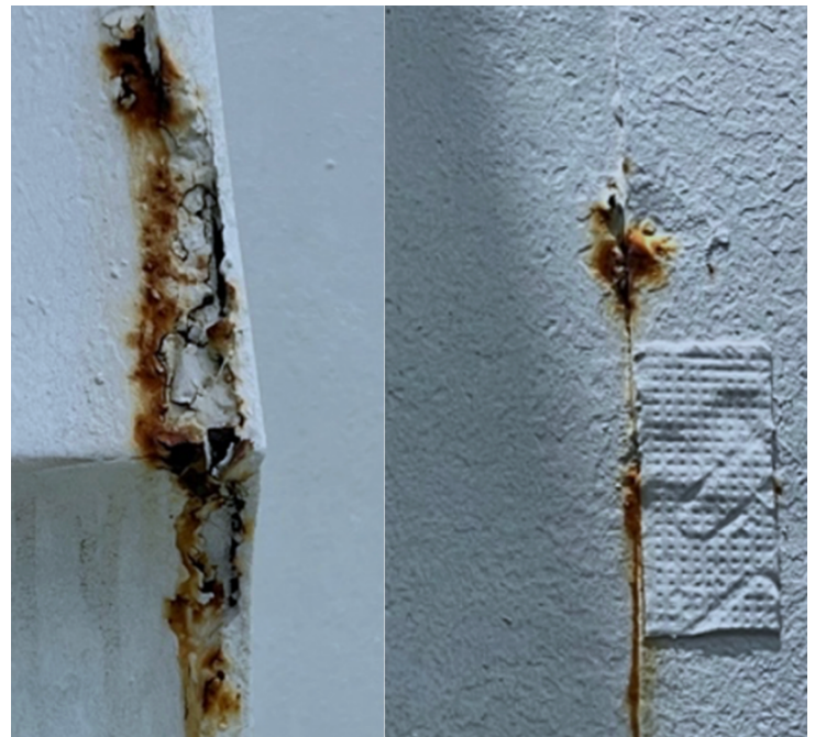
Examples of areas where tin cladding requires repair
