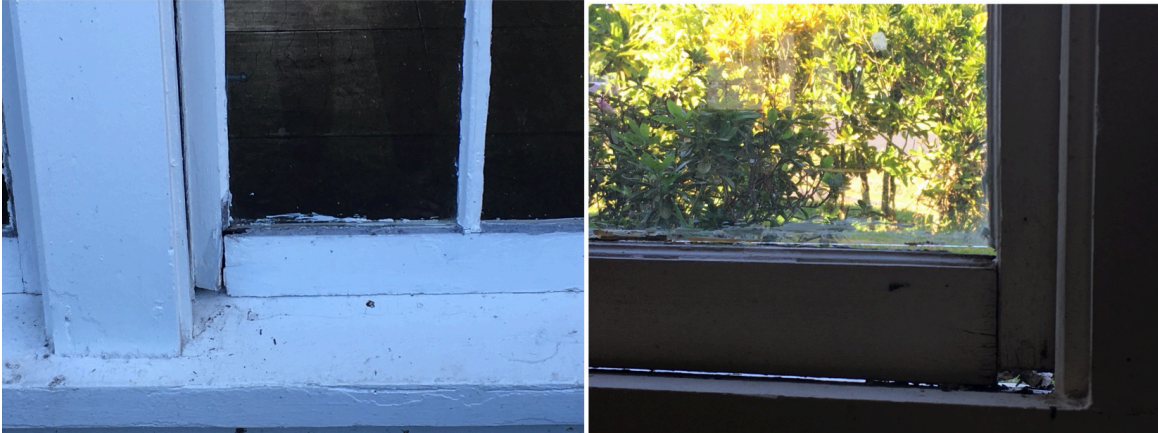
Social Hall windows are being rebuilt to insure they function well and maintain their structural integrity...they'll look better too!
