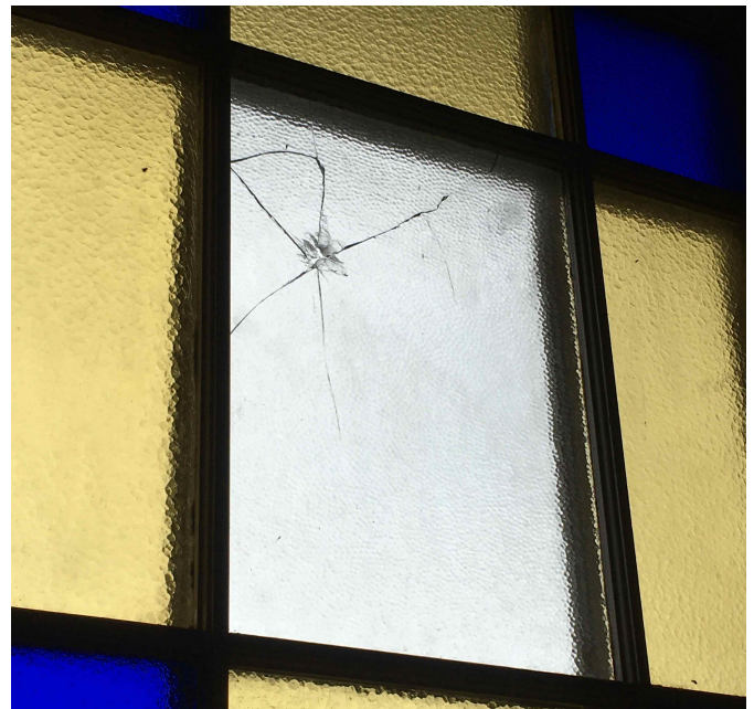
Multiple panes of art glass need replacing.
