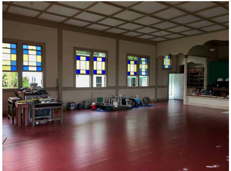
Almost done. Needed: completion of "punch list", clean up, and return of the pews.
